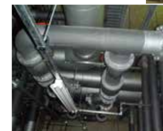
空調配管 Air conditioning piping system
