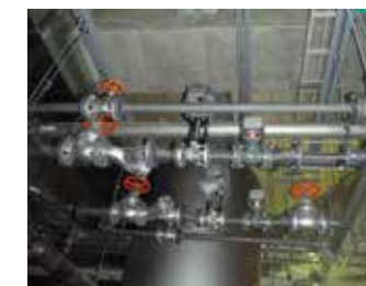
衛生用配管 Hygienic piping system
