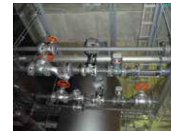
衛生用配管 Hygienic piping system
