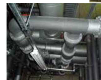
空調配管 Air conditioning piping system
