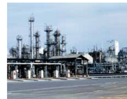
工場配管 Pipes for plant
