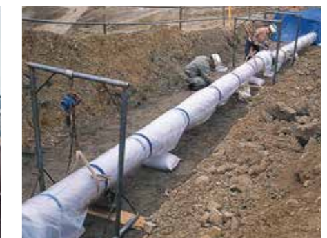
水道配水管 Water distribution / service pipes
